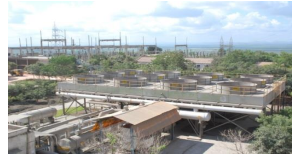
Waste heat recovery plant
