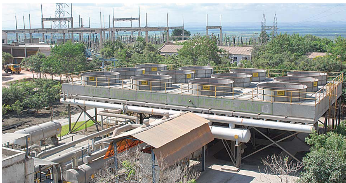
Conversion of waste heat into power at our Tadipatri plant
