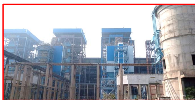
Dry Fly Ash conveying in silo through closed Pipelines
