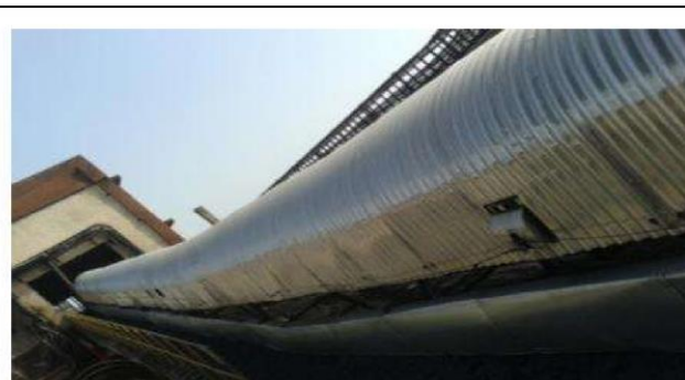
Coal Conveyor Belt closed
