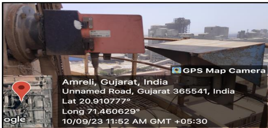
Opacity Meter installed at Stack
